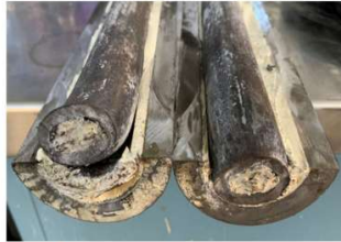
ON-12: Failure profile
