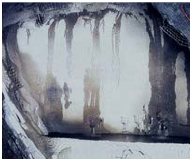
Figure 12 - Example of a shotcrete fill fence (source: Brunswick Mine, New Brunswick, Canada).
