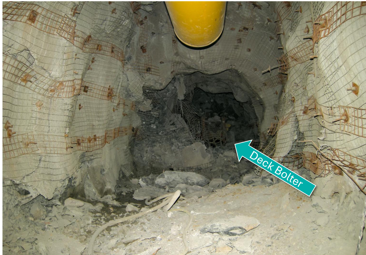
Seismic Damage in a Workplace from M_n 3.8 Seismic Event
