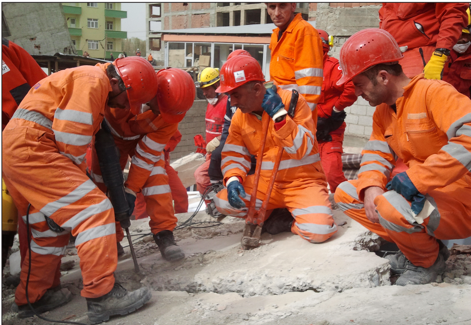
Jackhammers are not a standard piece of rescue equipment, but at least one Çayeli Mine Rescuer was so happy to have them available to dig through the concrete rubble of the Van earthquake, he offered to kiss them when the team returned home. Photos courtesy Inmet Mining
