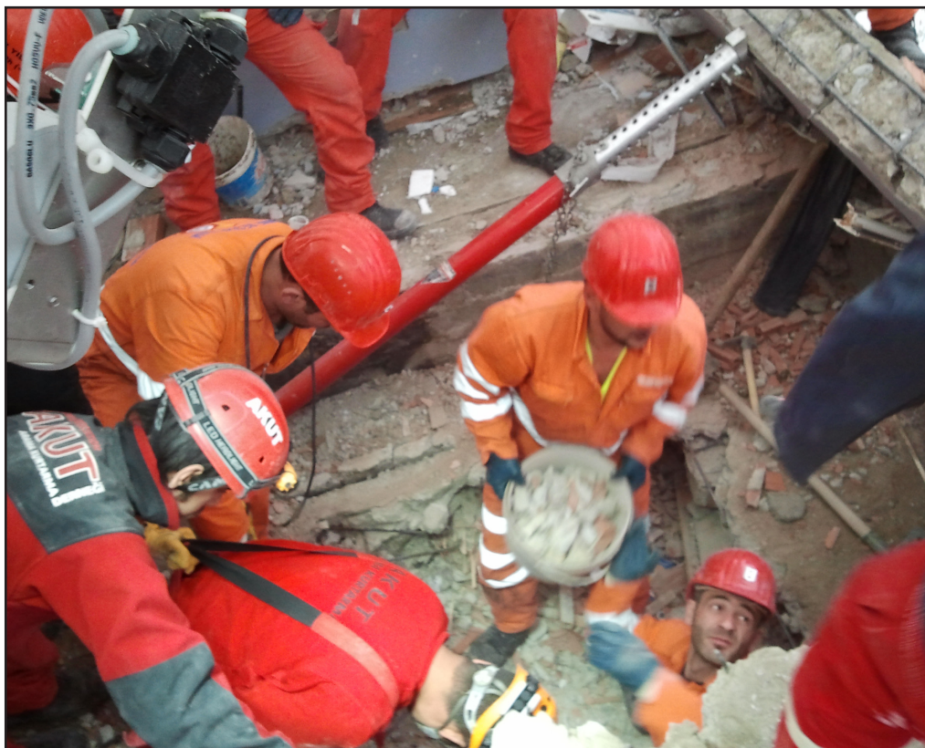
Mine rescuers from Inmet Mining's Çayeli mine remove rubble from a collapsed building following an earthquake in Van, Turkey. Photos courtesy Inmet Mining
