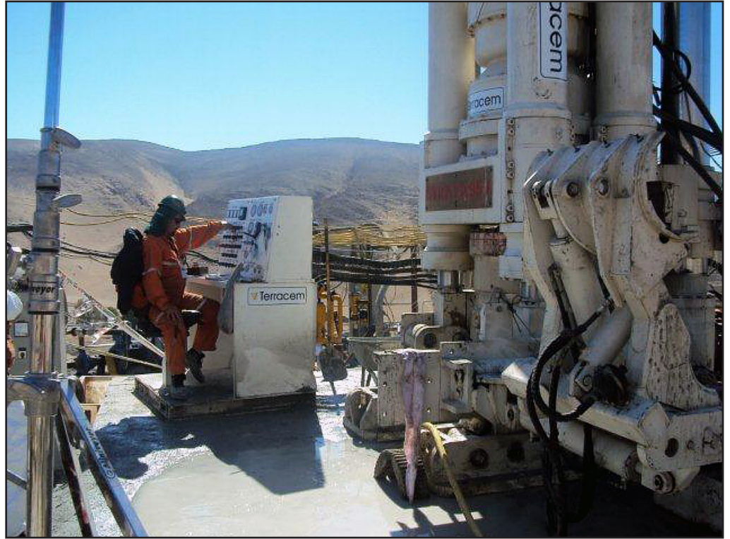
Cementation Canada’s Strata 950 raisebore, designed and manufactured by RUC Cementation in Australia, and operated by another Cementation Group company, Terracim, was a small part of a large international effort to save 33 Chilean miners.
